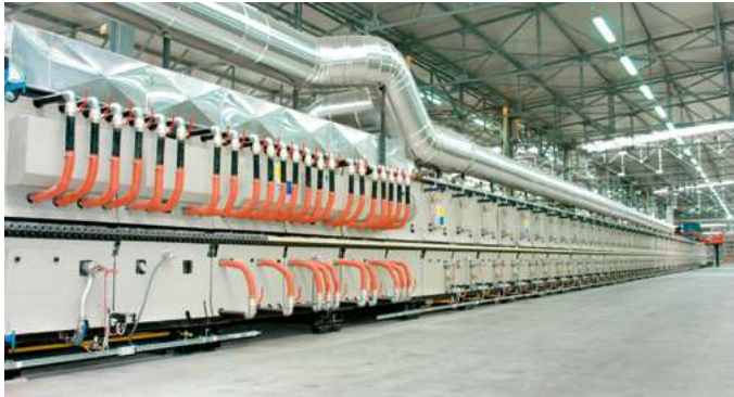
Roller hearth furnace
