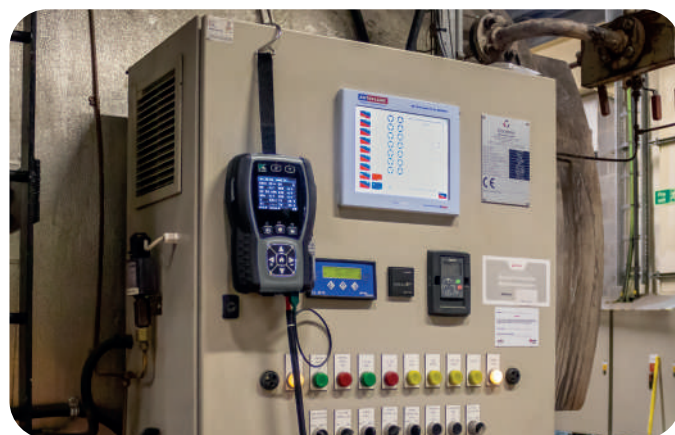
Testing boiler emissions
